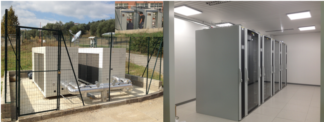
Figure 1: (Left) The two-Chiller system (with integrated free cooling) installed at the ReCaS Cosenza Site. (Right) The white space and the racks (with LCPs) hosting part of the IT equipment.
