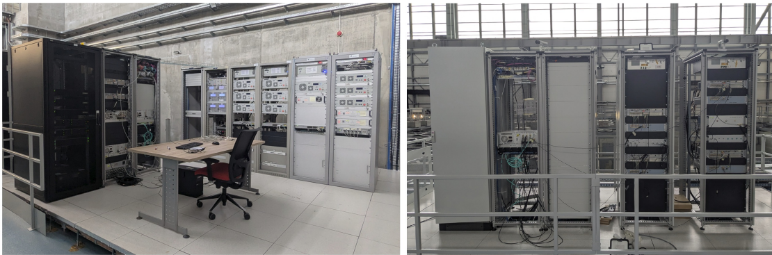
Figure 6: Racks in the "Corridor" area (left) and "roof" area (right).
