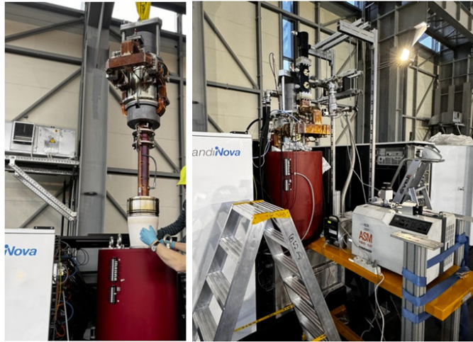
Figure 3: Klystron installation in the modulator (left); vacuum test of the high power rf load installed at the klystron waveguide output (right).
